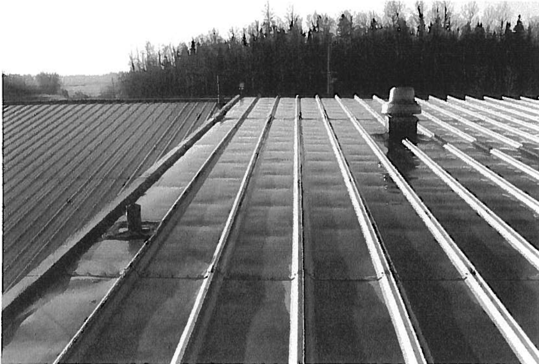
View of original City Garage roof looking south: note two (2) seams and Fire Hall addition to the east (left).
