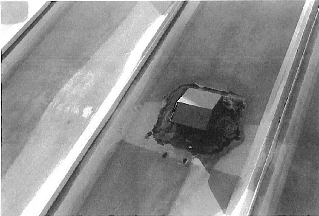
Existing roof penetration to be re-flashed: exhaust fan
