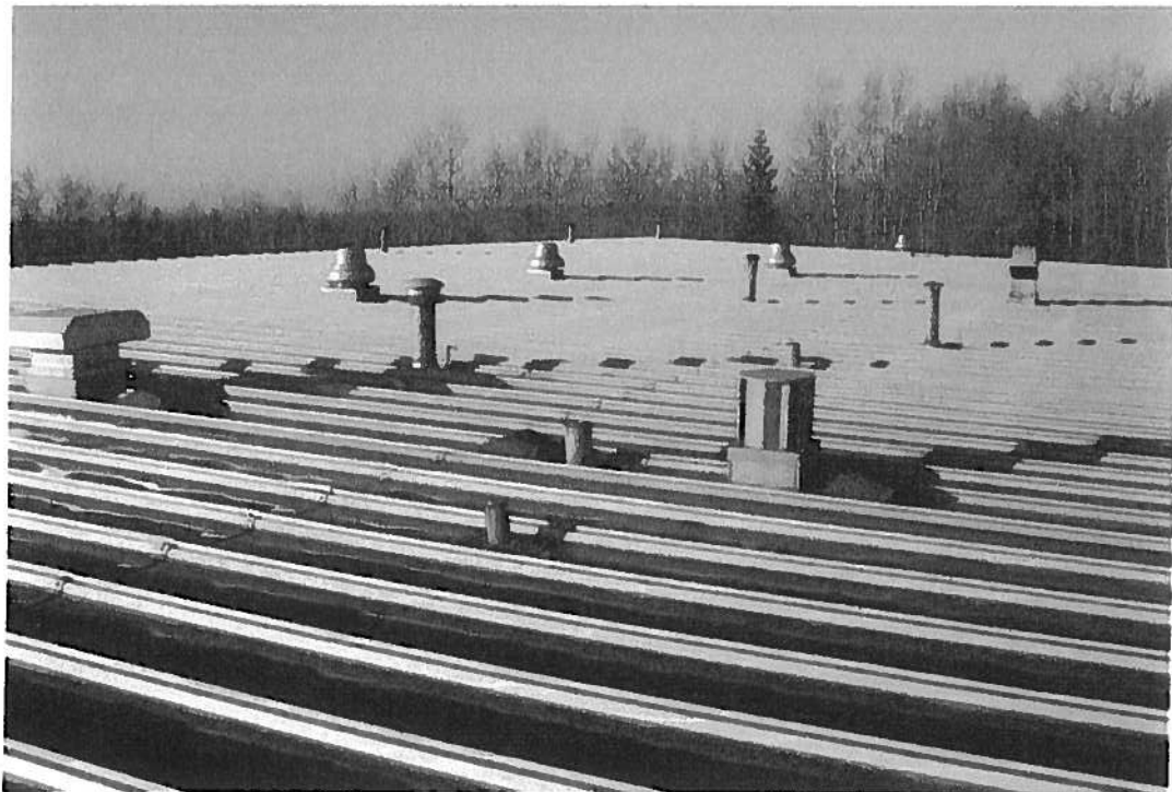
View of existing City Garage roof: note 21 roof penetrations to be re-sealed.
