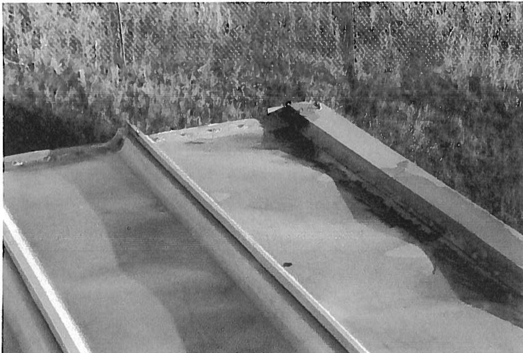
Roof edge at east and west to be re-flashed.
